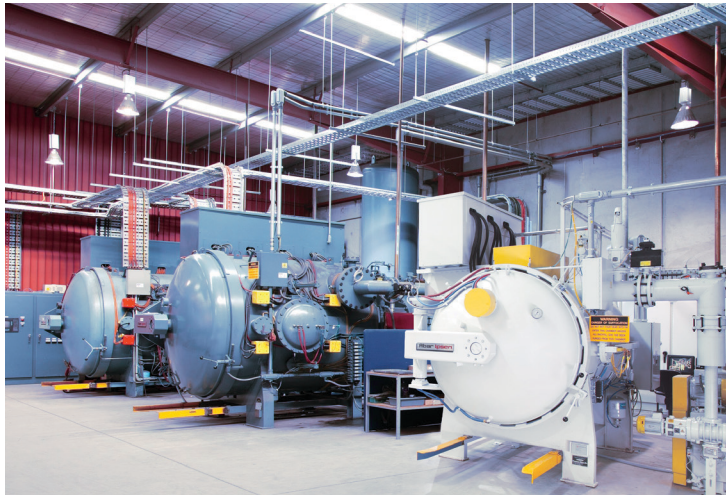
Vacuum Furnaces inside the Surface Technology Coatings plant
